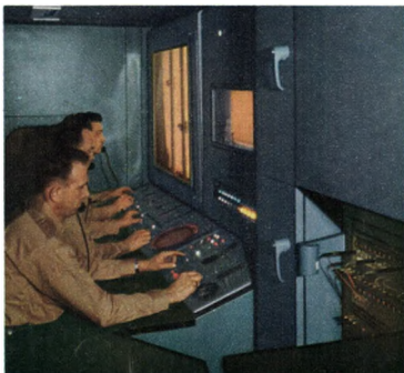
Inside central control van, these soldiers watch radarscopes as Nike automatically guides a missile to its target.
