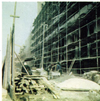
Construction in Minsk. City was 75 per cent wrecked by Nazis, is being rebuilt wholesale
